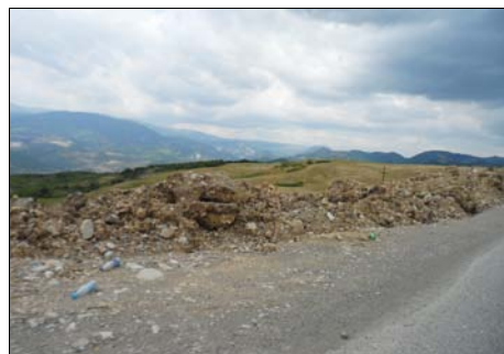
Picture 2. The road section on the 76th km of the Baku-Shemakhy highway is destroyed, 2018.
